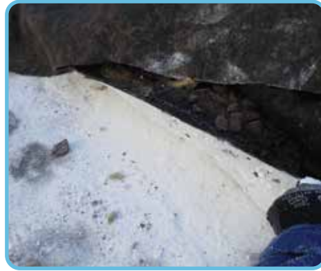
All the contaminated layers were removed until the clean Oilmat and Albasorb could be seen.
