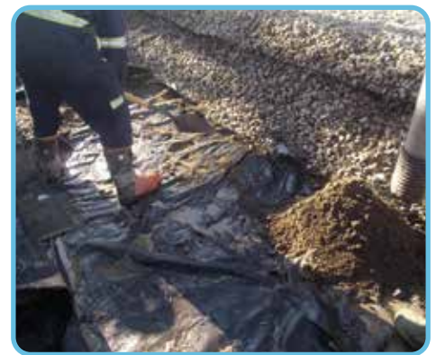
The top contaminated sand layer was removed within the contamination area using the Vac-truck.
