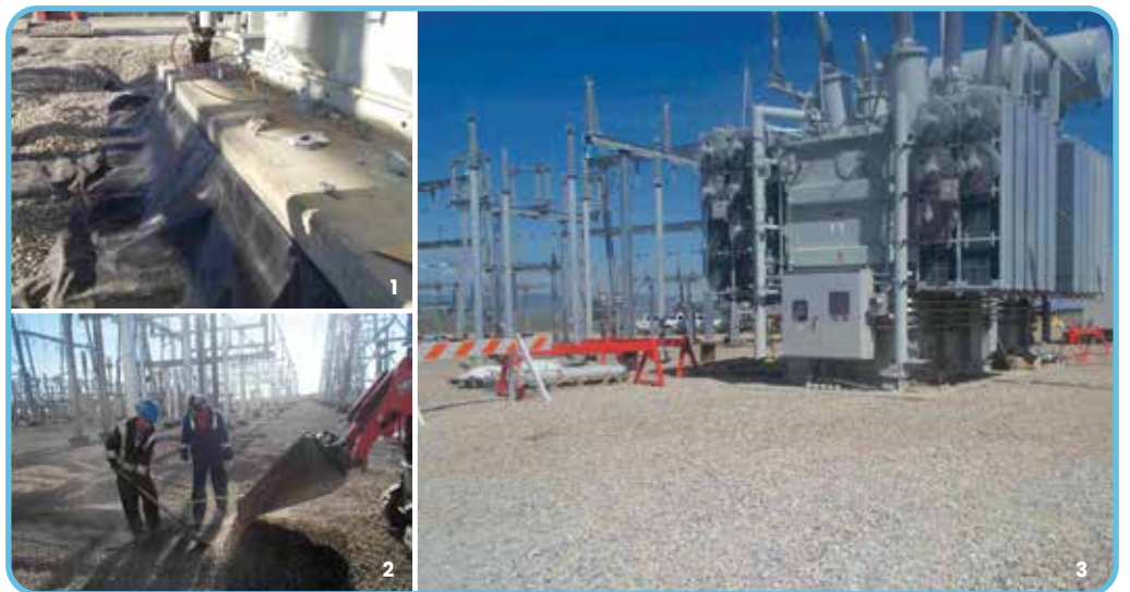
1. The sand beneath the congealed oilmat was observed to be clean and unaffected by the spill. 2. Stone was replaced in the affected area. 3. The site was cleared of all debris and all equipment was removed from the substation.
