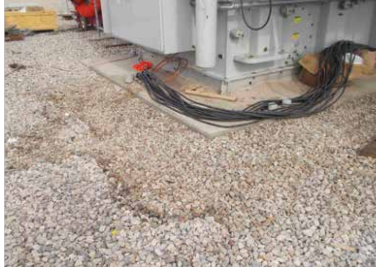
Visual discoloration was observed from the area that came into contact with the oil.
