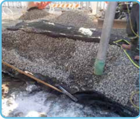
The construction crew removed and disposed of all the layers that came into contact with the oil.
