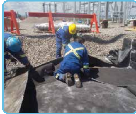
A new Oilmat was cut and placed, maintaining the required minimum overlap in between the existing and new Oilmat layers.
