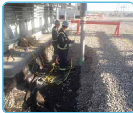
The existing non-woven geotextile showed signs of oil contamination, which was removed and discarded.
