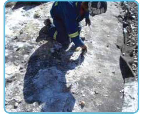
The contaminated Oilmat was removed and disposed of by the construction crew.
